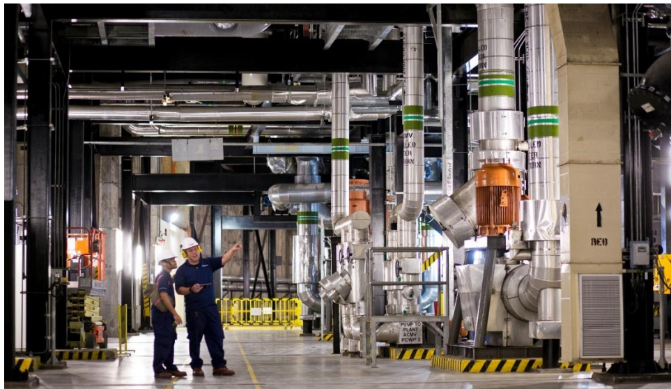
SP Group operates one of the world's largest underground district cooling system that supplies chilled water for air conditioning to buildings in the Marina Bay area with connected buildings enjoying up to 40% energy savings.
