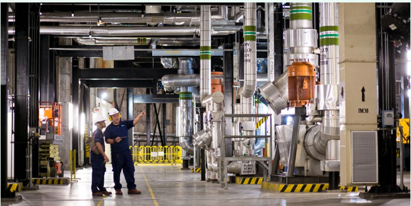
SP Group operates the world's largest underground district cooling system that supplies chilled water for air conditioning to buildings in the Marina Bay area.
