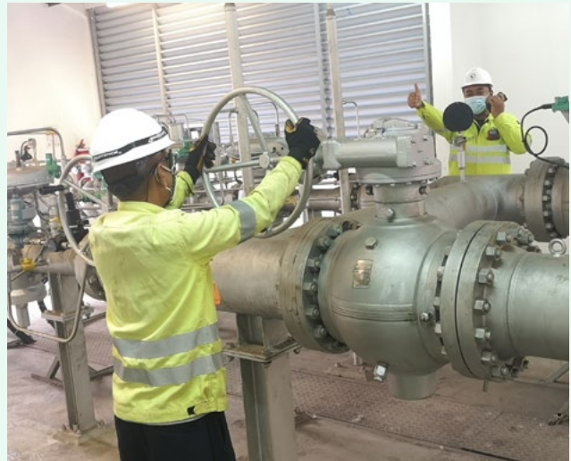
SP Group checks the gas regulators regularly to ensure optimal gas supply pressure for customers.
