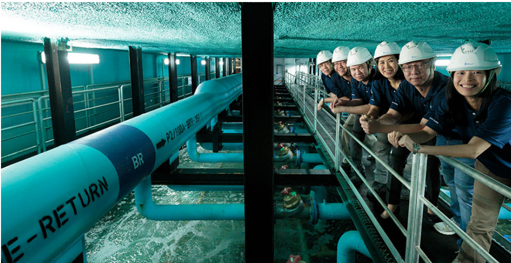
Bottom: SP Group's district cooling system at Marina Bay.
