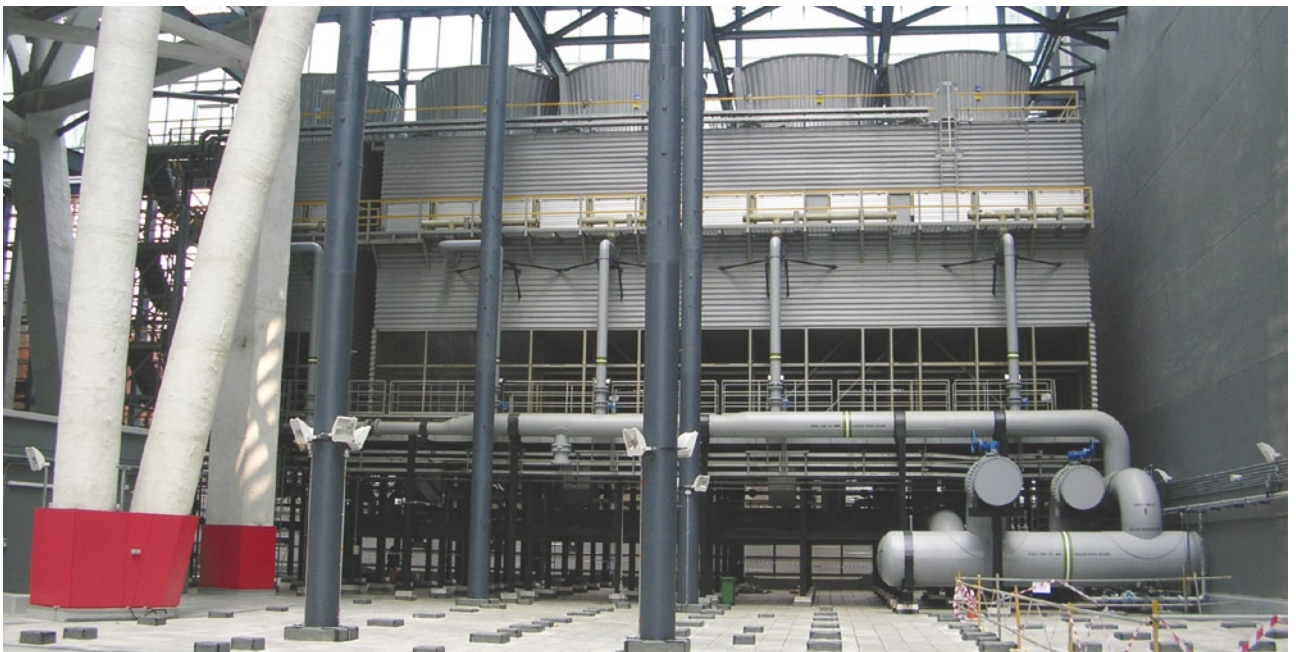
A centralised cooling tower eliminates the need for an in-house chiller plant in buildings.
