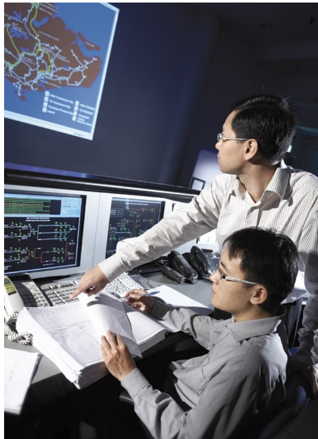
A sophisticated Supervisory Control and Data Acquisition system lies at the heart of PowerGas' operations.
