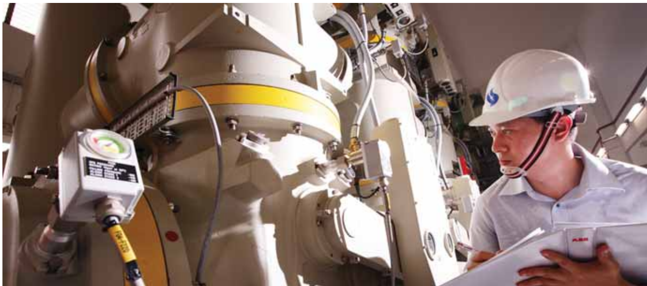
An engineer checks a 66kV switchboard
