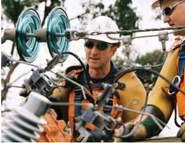
SPI (Australia) Assets operates major electricity distribution assets in Melbourne and southeast of the city
