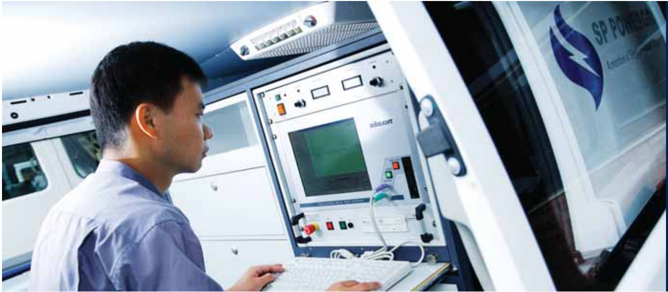
The cutting-edge Oscillating Wave Test equipment helps engineers monitor the condition of cables
