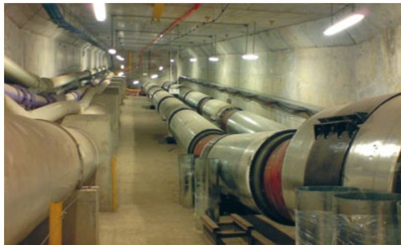
Installation of a new piping network in the Common Services Tunnels will link the district cooling plants and customer intake stations.
