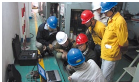
SP PowerGrid engineers conducting Condition Monitoring tests in Guangzhou, China.
