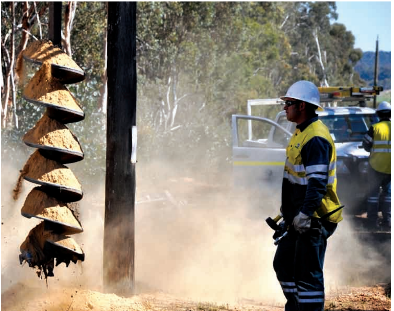
Jemena continues to deliver safe and reliable infrastructure services to asset owners throughout Australia.
