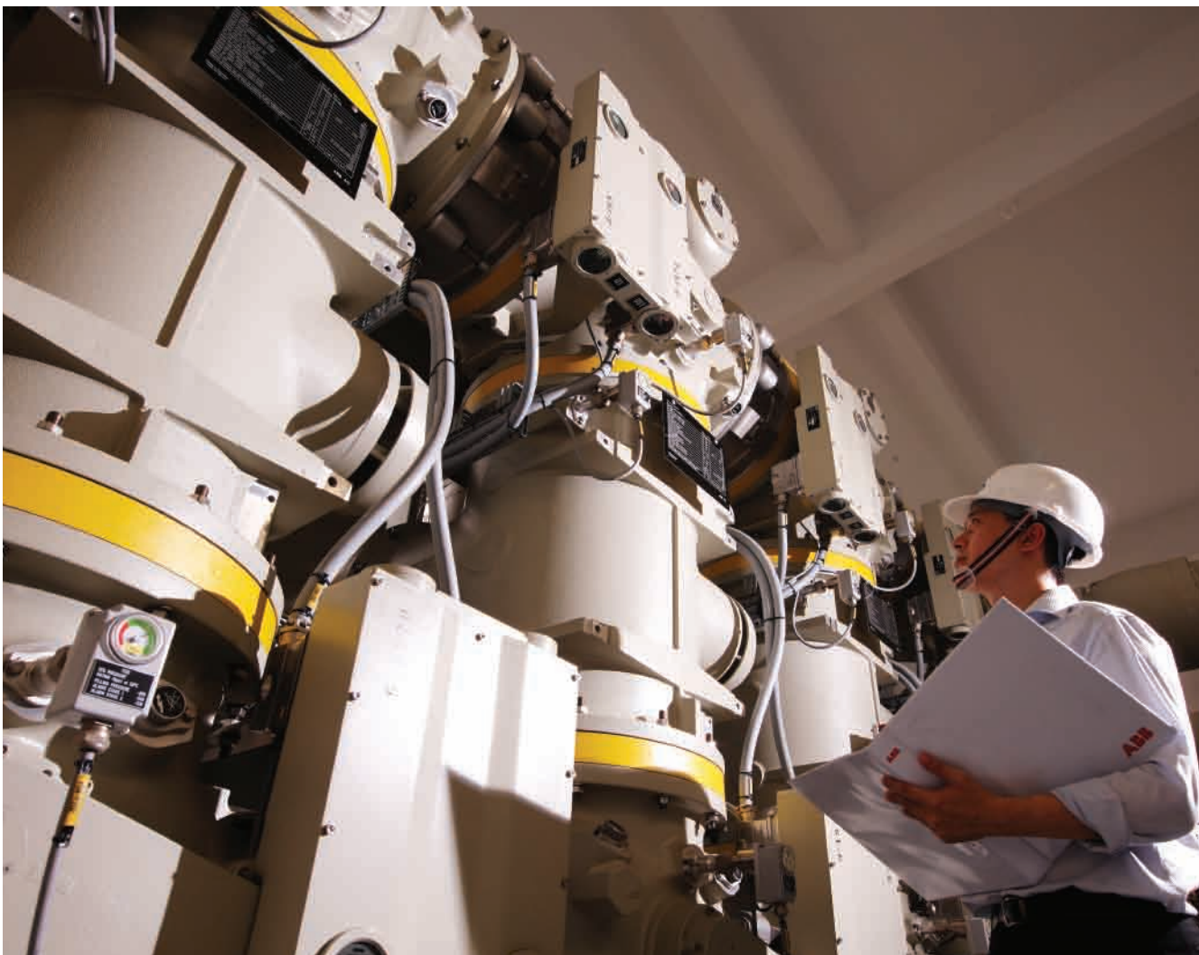
An engineer checking a 66kV switchboard.
