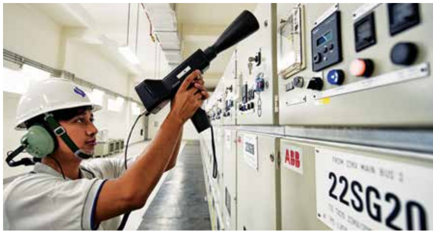
Condition monitoring detects and removes incipient faults to help avert network failure.
