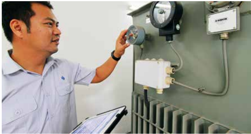
The substation inspection mobile app allows inspectors to carry out their work more efficiently.
