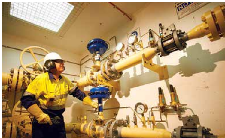
A Zinfra Group operator checking the pressure control valve at a gas distribution station in the MultiNet Gas network.
