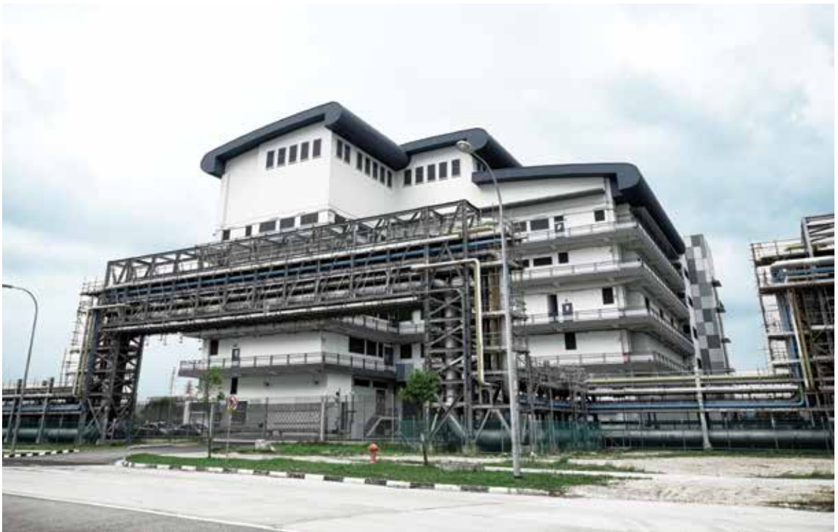
The Tembusu 230/66kV Substation is the first in Singapore to be installed with 500MVA 230kV series reactors, which will reduce the fault currents in the network and increase power resilience.
