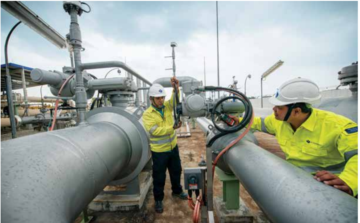
Technical Officers Mohamed Musa bin Abdul Majeed (left) and Yakob Bin Mahdar carrying out inspection works at the Banyan gas offtake station.
