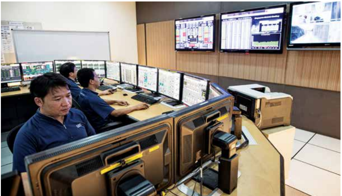
Staff at Singapore District Cooling work round the clock to deliver high levels of performance and reliability for customers.
