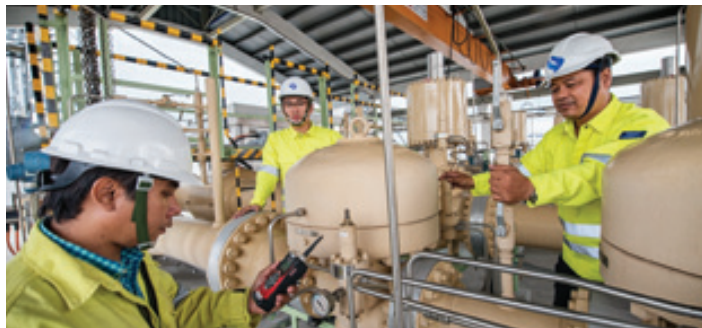
From Left: Gas Transmission Projects Technical Officer Mohamed Musa bin Abdul Majeed, Executive Engineer Lian Junyue, and Technical Officer Yakob Bin Mahdar preparing to carry out equipment maintenance works at an off-take station
