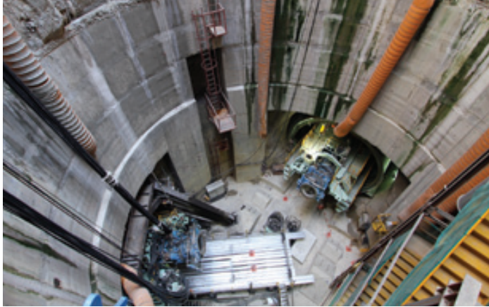
For the construction of the cross-island cable tunnel, the tunnel boring machine excavates through soil and rock strata underground
